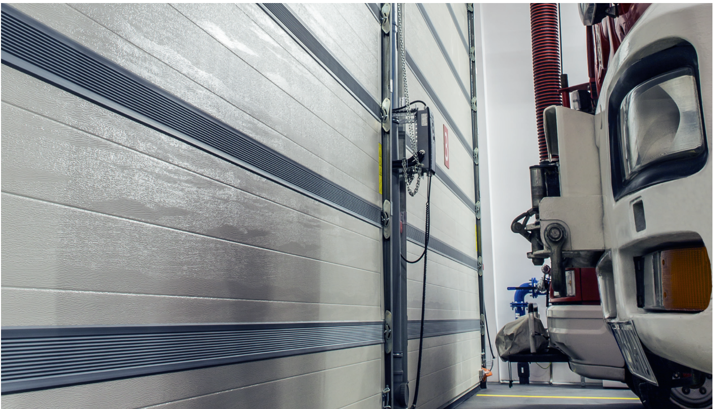
MakroTherm 2.0 doors (as seen from the inside).
